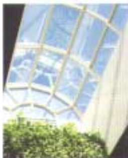
An unprotected skylight.
